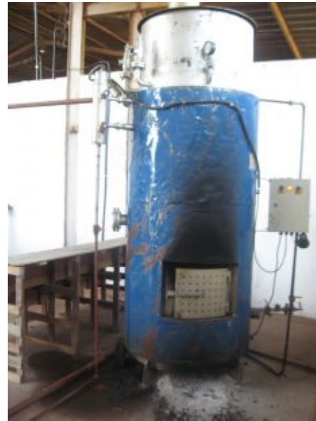
Figure 6.32: Autoclave from the side
